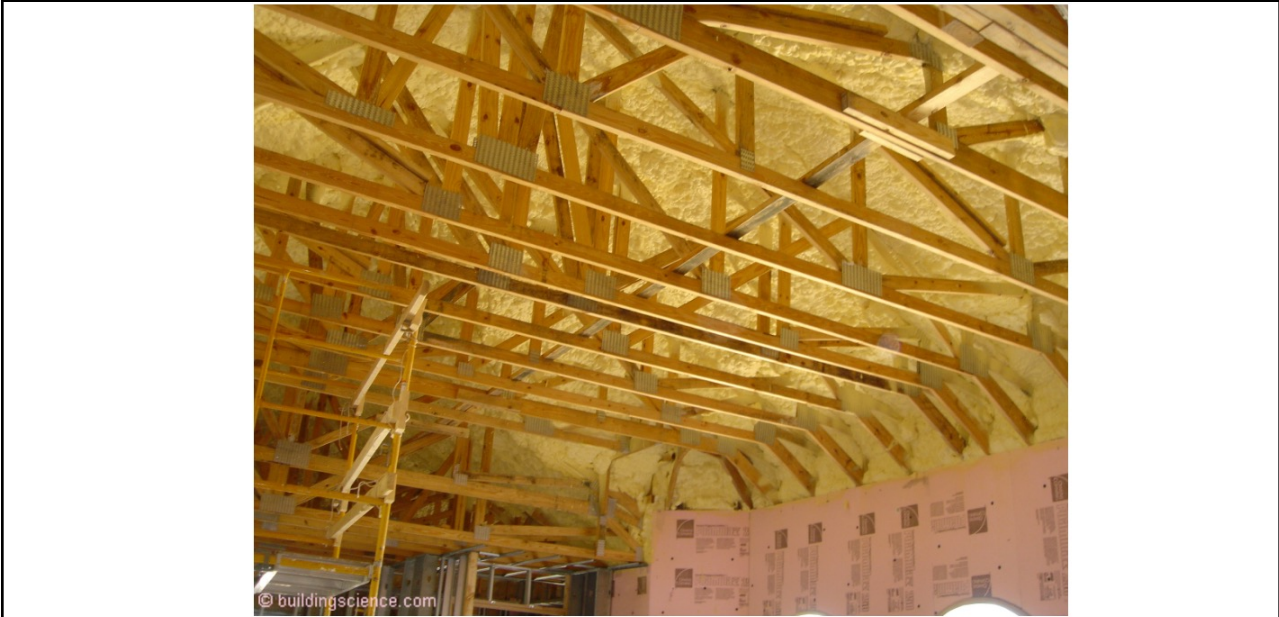
Photograph 8: Open Cell Spray Polyurethane Foam (ocSPF) - When you spray ocSPF into wall cavities from the interior the ocSPF can act as the air control layer and thermal control layer. It can't act as the vapor control layer - it is too vapor open. This is a problem when you spray ocSPF on the underside of roof/attic assemblies you can end up with problems ("Ping Pong Water").
